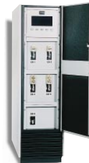
Fig. 7 Static Transfer Switch rated 200 amperes.
