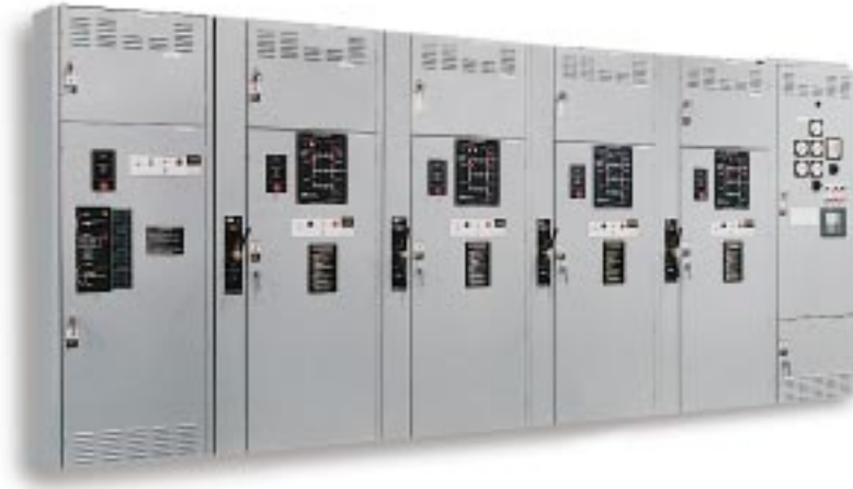
Fig. 15 ATS Switchboard with five automatic transfer bypass isolation switches, and emergency distribution circuit breakers.
