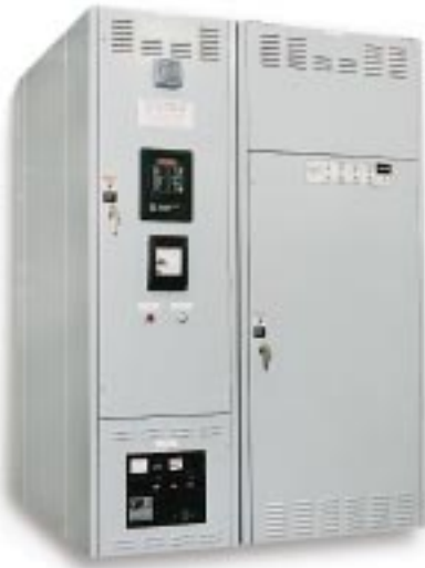
Fig. 11 Two source system with main circuit breaker, protective relaying and and Automatic Transfer Switch rated 1200 amperes.
