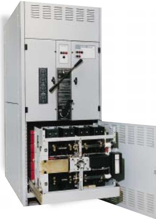
Fig. 3 Automatic Transfer & Bypass Isolation Switch rated 4 pole 2000 amperes.
