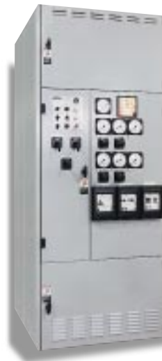
Fig. 5 Soft Load Closed Transition Transfer Switch rated 3 pole 800 amperes.
