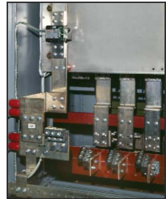
Fig. 16: Rear views showing ground fault protection with ground and neutral disconnect links
