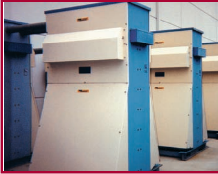
Installed 375 KVAR units (model K841) can be used individually or in parallel depending on load requirements.
