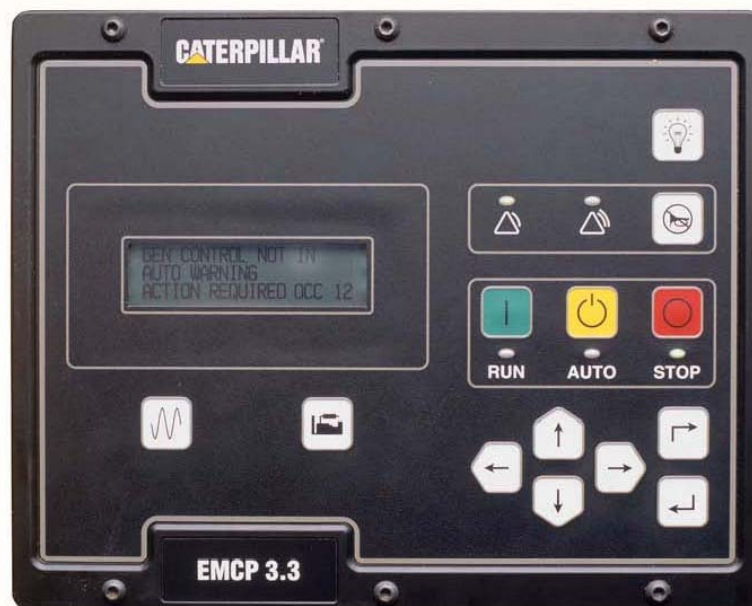
Fig. 4.1. EMCP3.3 Local control panel
